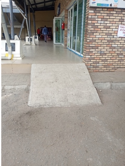
Figure 8. 1200mm wide ramp with 7° slope angles positioned without handrails, and signage (Source: Authors).
